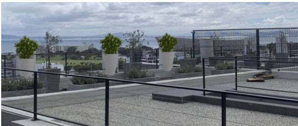
Base telecommunication stations
